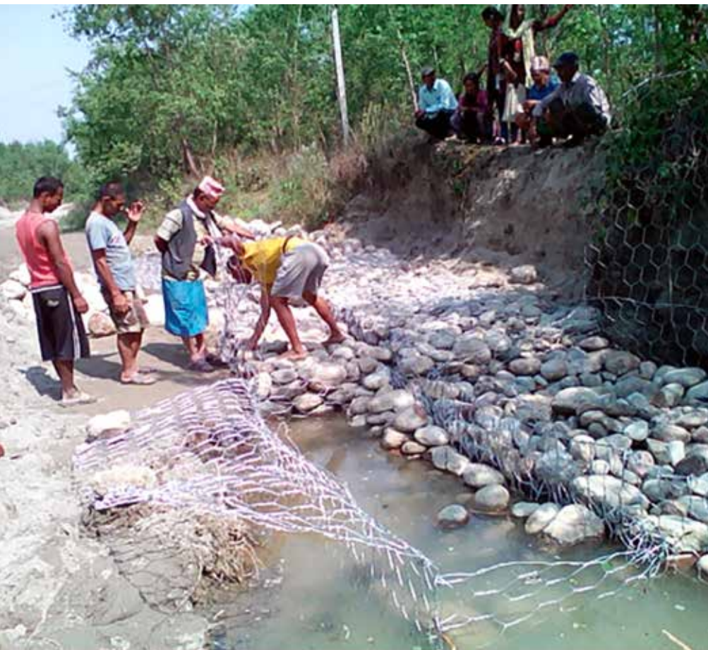
NEPAL: Riverbank stabilization project in Nepal to address increased erosion. One aspect of this project is that it uses locally-available materials. Another is that the project improvements can be maintained locally.
